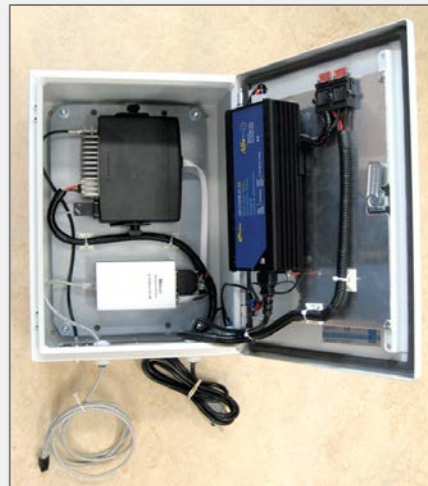
Above: Radio and interface built into a wall cabinet.
